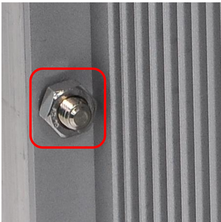
Ground screw of the switch
