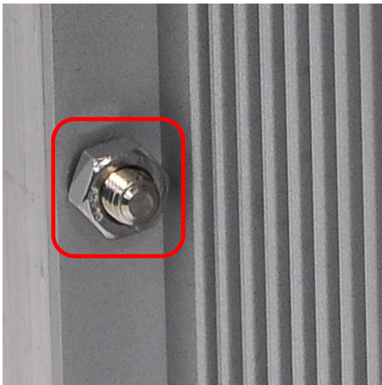
Ground screw of the switch
